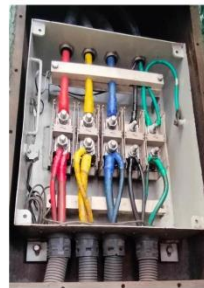
Junction box (Type-III) New RCF design
