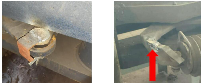
Fig 7-Wrong welding of APD
