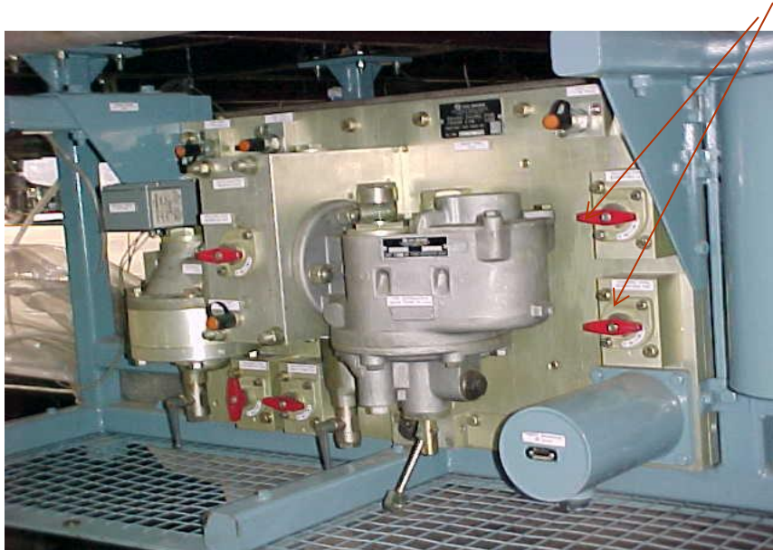
FTRIL CONTROL PANEL
